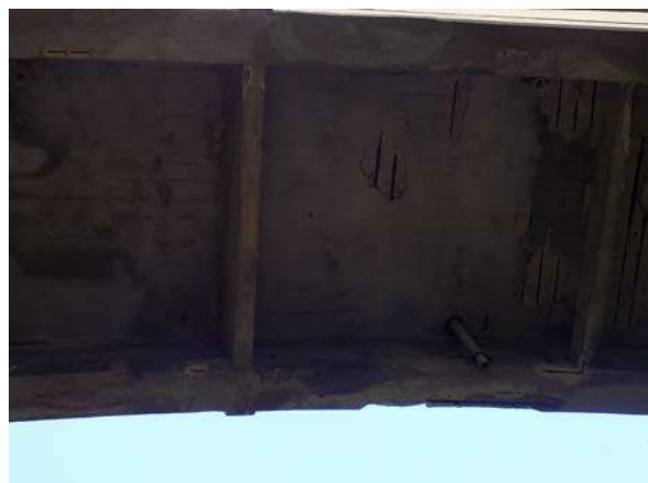
Photo 3: Underside of deck with delaminations
