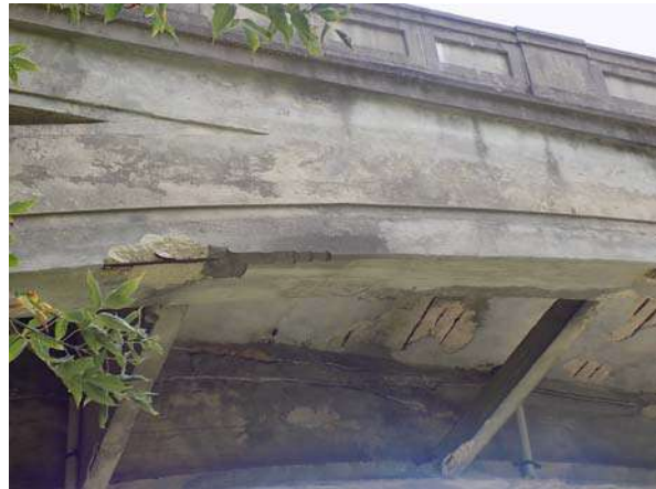
Photo 2: Corner spalls with exposed reinforcing steel on the arch rib
